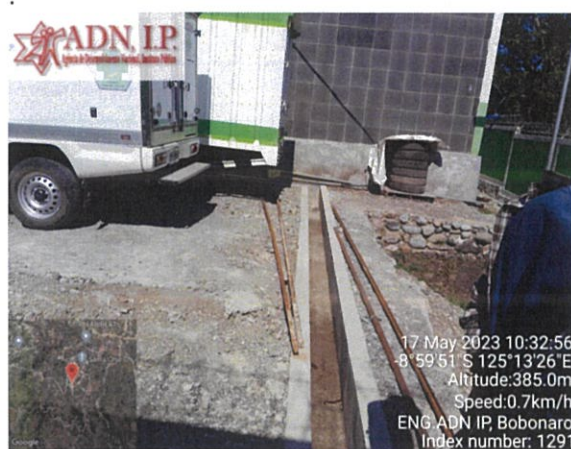
Foto : Wall plester internal drainage.
