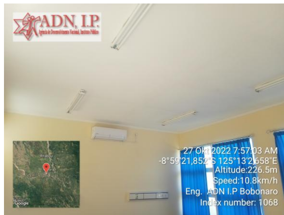
Foto : Supply and install Air conditioner Panasonic 2 Pk + all accessories
