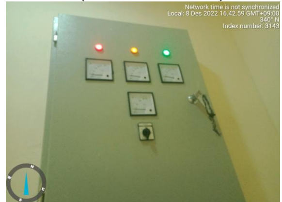
Foto : Supply & install Distribution Panel board LVMDP 900x700x250, External + all accessories (Inc.Connect to EDTL)
